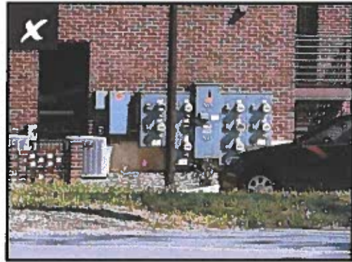
Mechanical Equipment Not Screened
