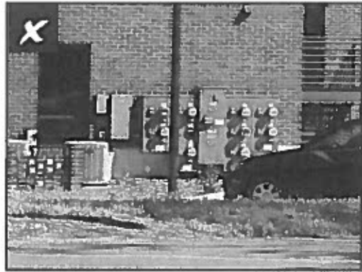
Mechanical Equipment Not Screened
