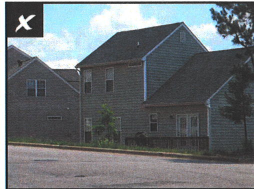
Less than 9-inch Overhang
