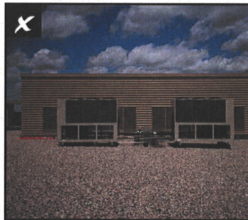
Unscreened Roof-top Equipment
